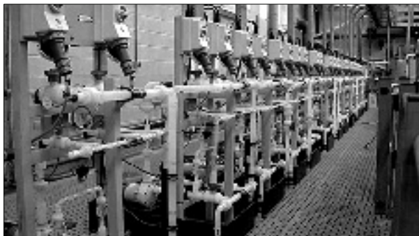
Figura 1 – Distribuzione acqua con condotte in PVDF Figure 1 – Hook up piping system out of PVDF for water
